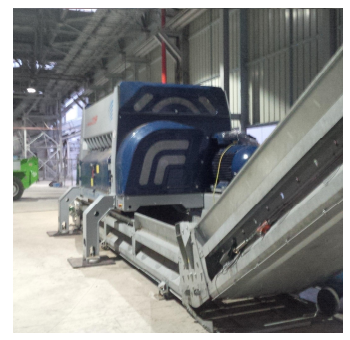
SECONDARY SHREDDER TO ADJUST THE SRF TO THE REQUIRED SIZING SPECIFICATIONS
