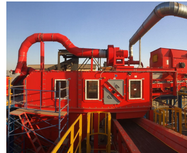
AIR SEPARATOR, TO SEPARATE HIGH QUALITY FRACTION, FROM MATERIAL WITH LOW CALORIFIC POWER
